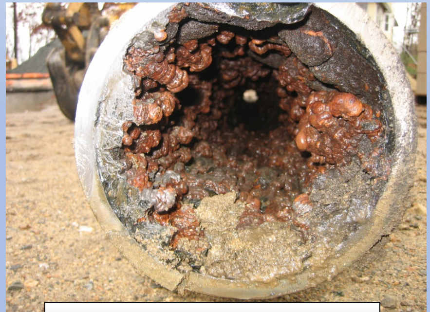
80 Year Old Unlined Water Pipe
