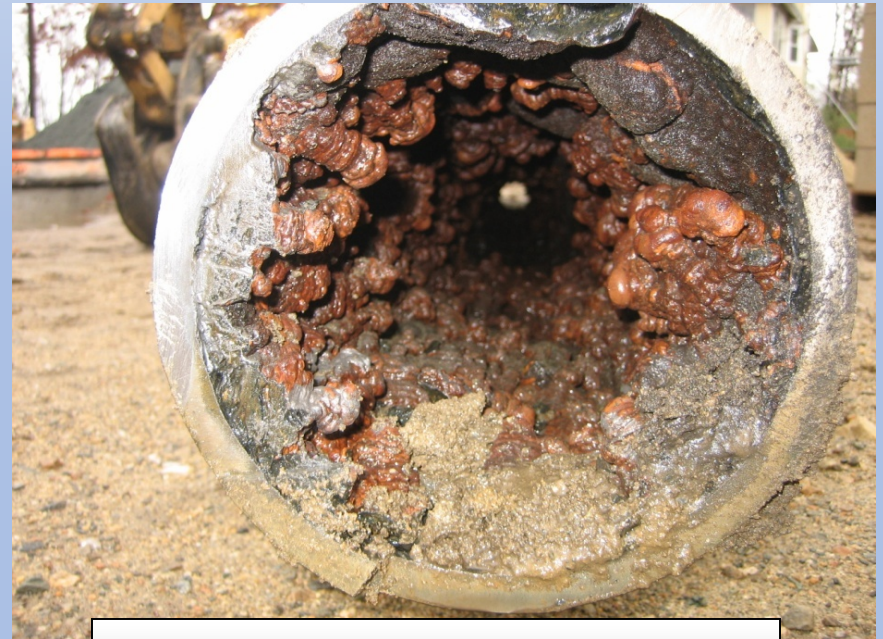
80 Year Old Unlined Water Pipe
