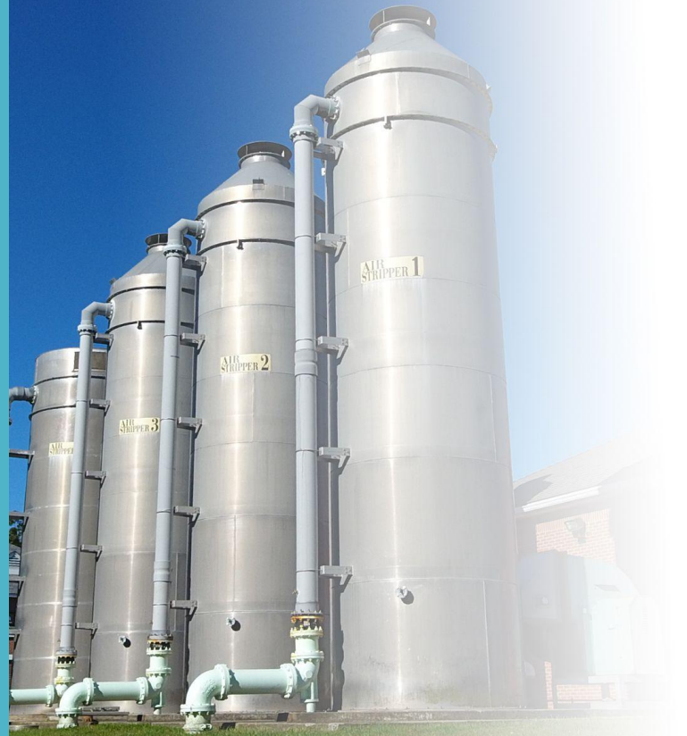
Air Stripping process for VOC treatment at Springvale Treatment Plant
